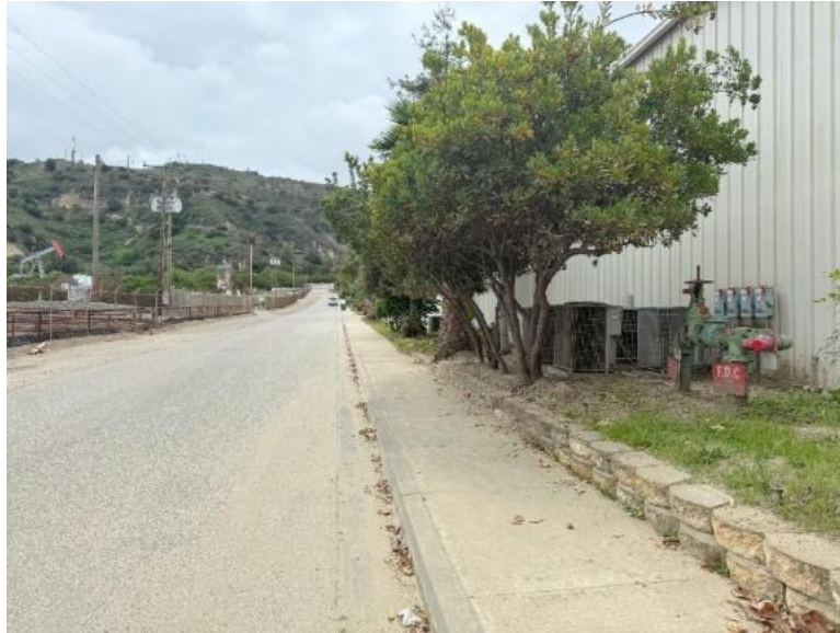
Exhibit 3-31: Fire department connection on the south side of Ventura Steel Site
